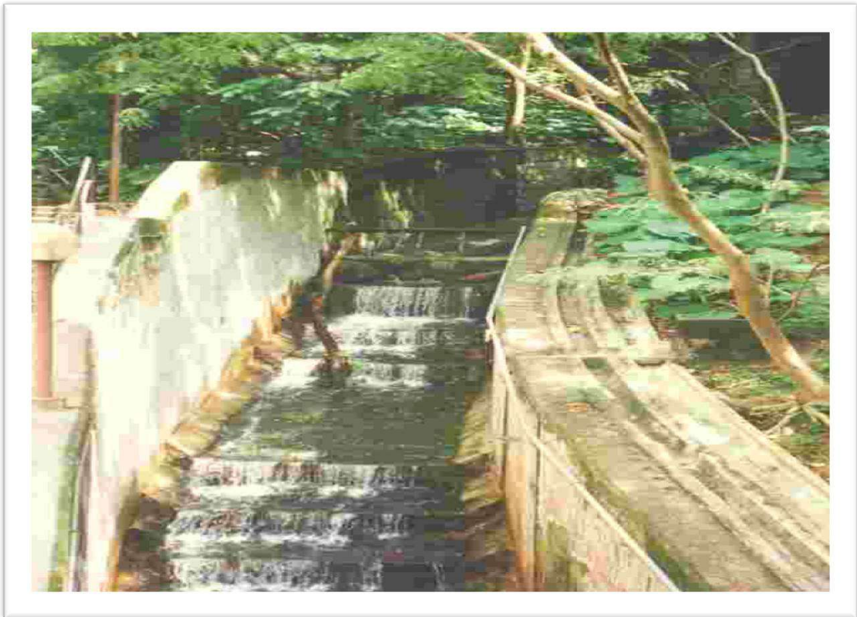
Figure 1.7 Stepped storm water beneath the University of Hong Kong
