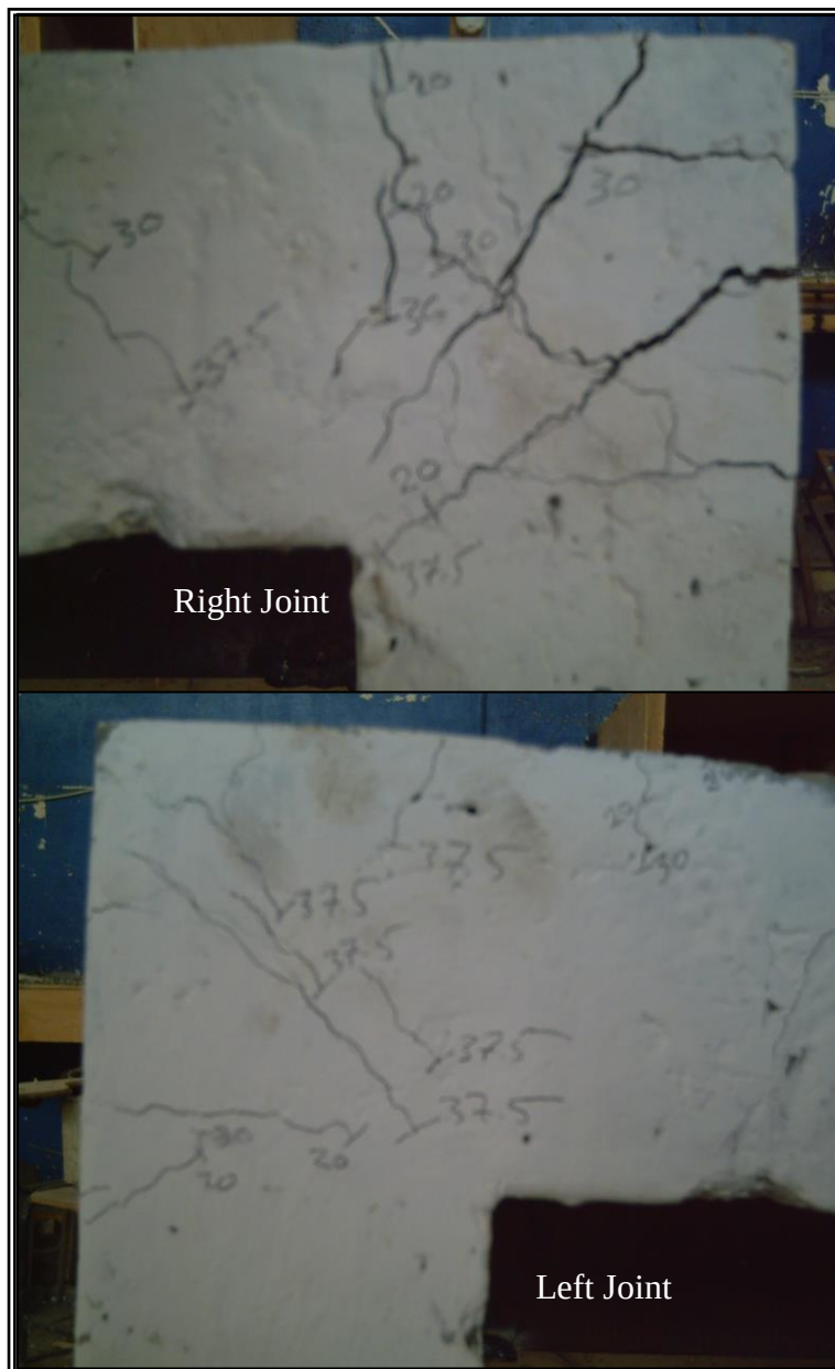
Figure (6.8) Joint Failure of FRAME2
