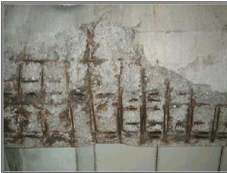
Figure (1.1): Corrosion of Reinforced Concrete Member
