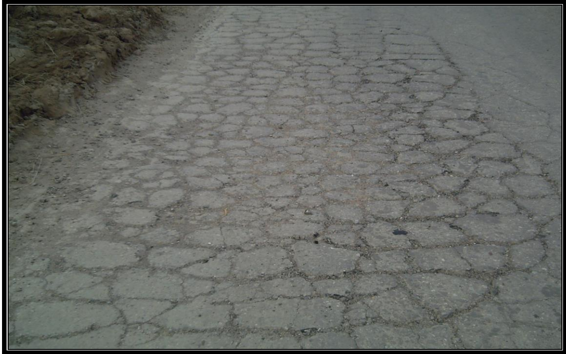
Figure (2-3) Fatigue Cracking
