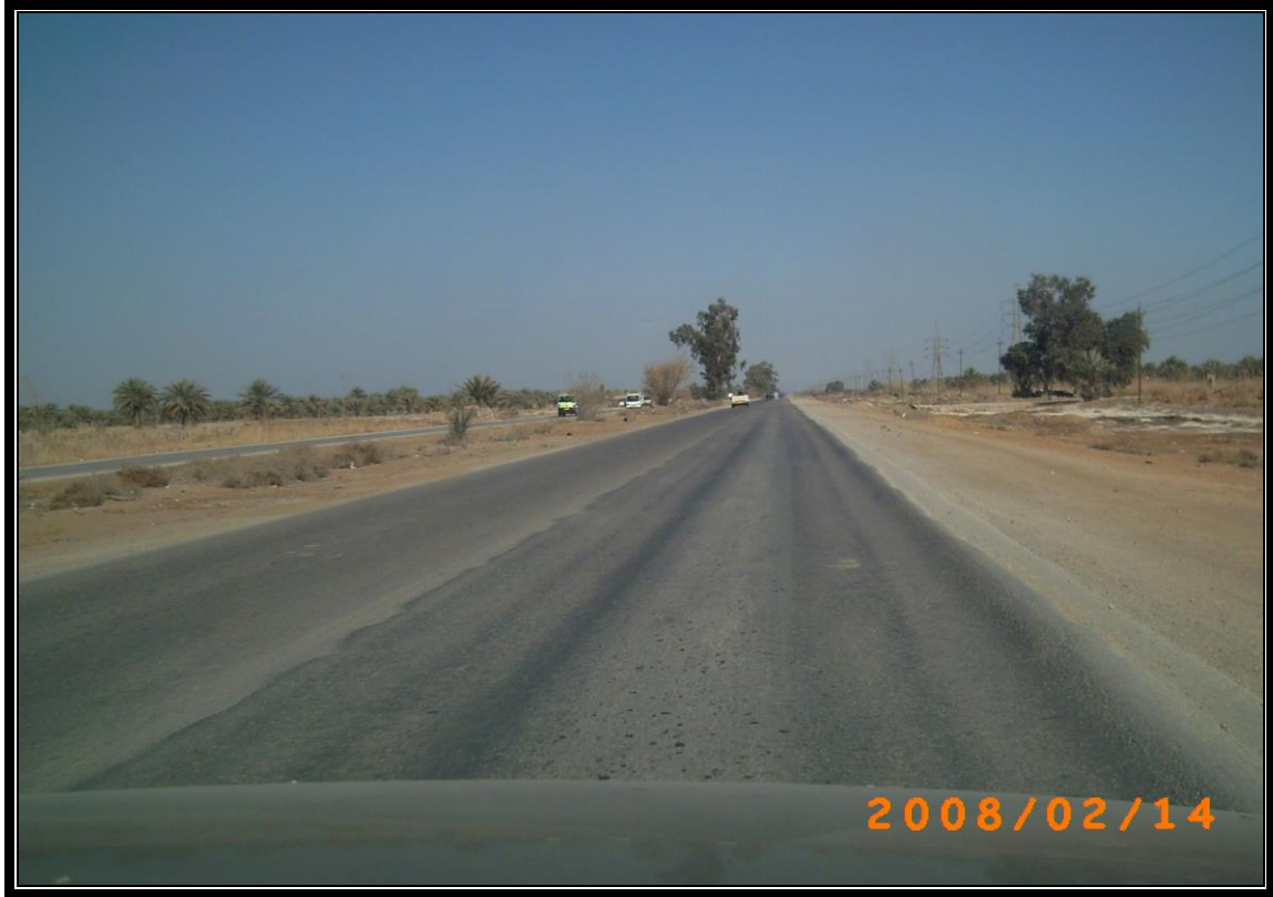
Figure (2-6) Pavement Rutting
