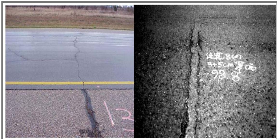
(a) Traditional Single Reflective Cracking (b) Double Reflective Cracking
