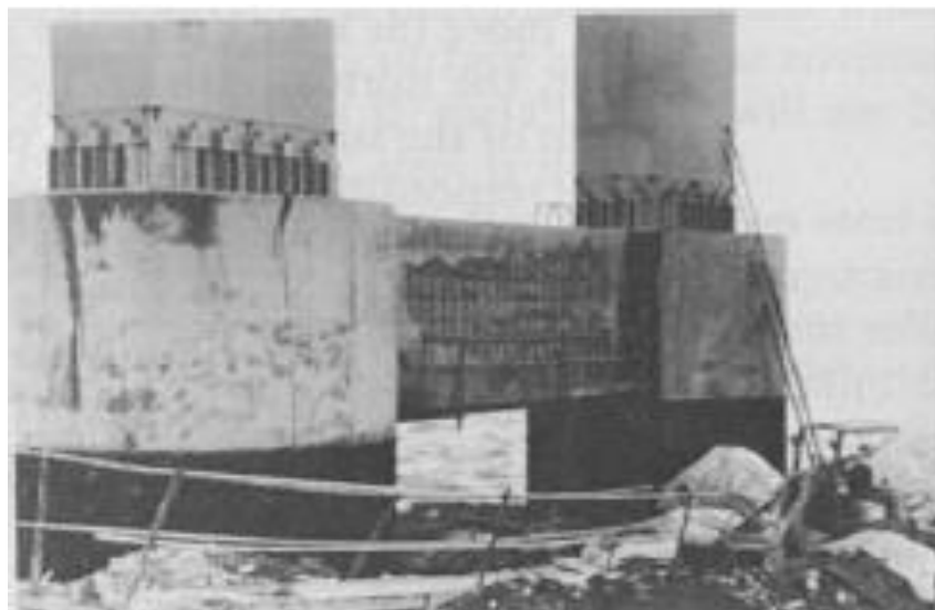
Plate (1-2) Damage to reinforced concrete structures due to corrosion of steel [16].
