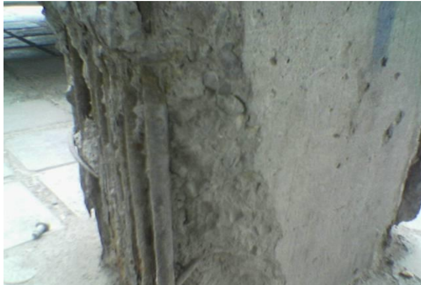
Plate (1-1) delaminating of cover due to corrosion
