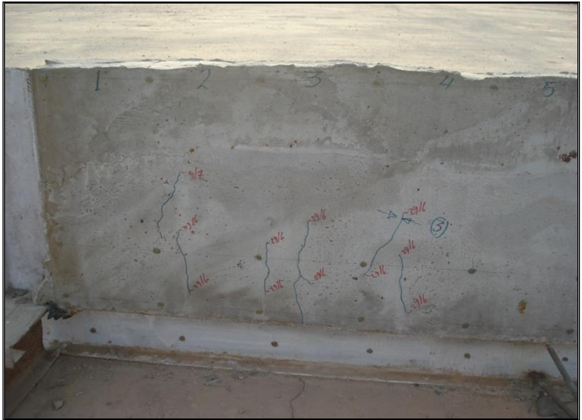
Plate (4-1) Final cracking pattern of first quarter of wall (8S)
