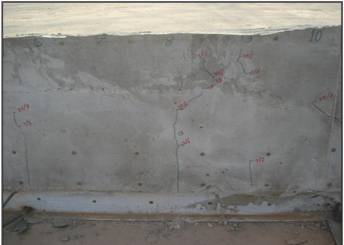
Plate (4-2) Final cracking pattern of second quarter of wall (8S)
