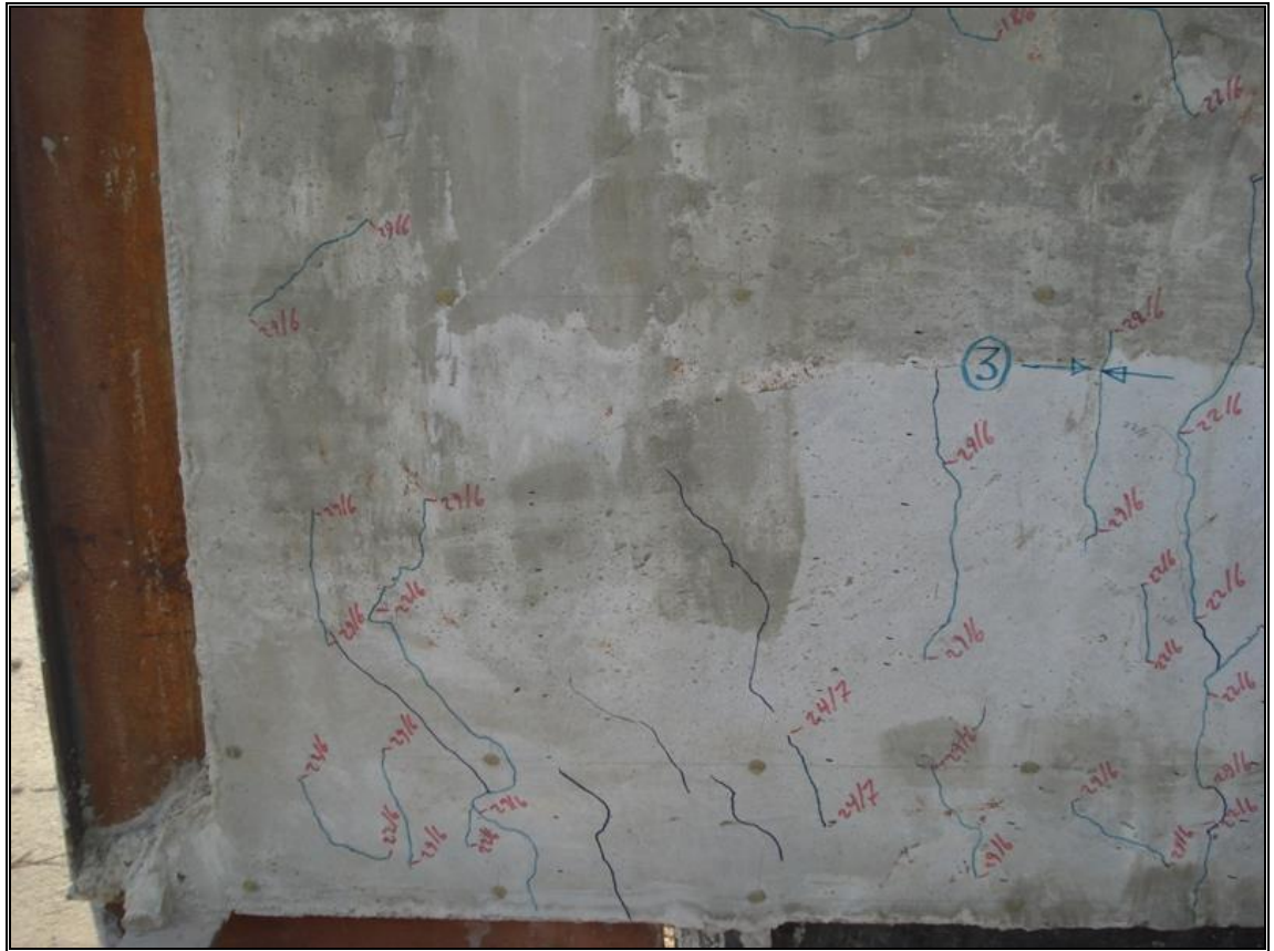
Plate (4-9) Final cracking pattern of first third of wall (2S)
