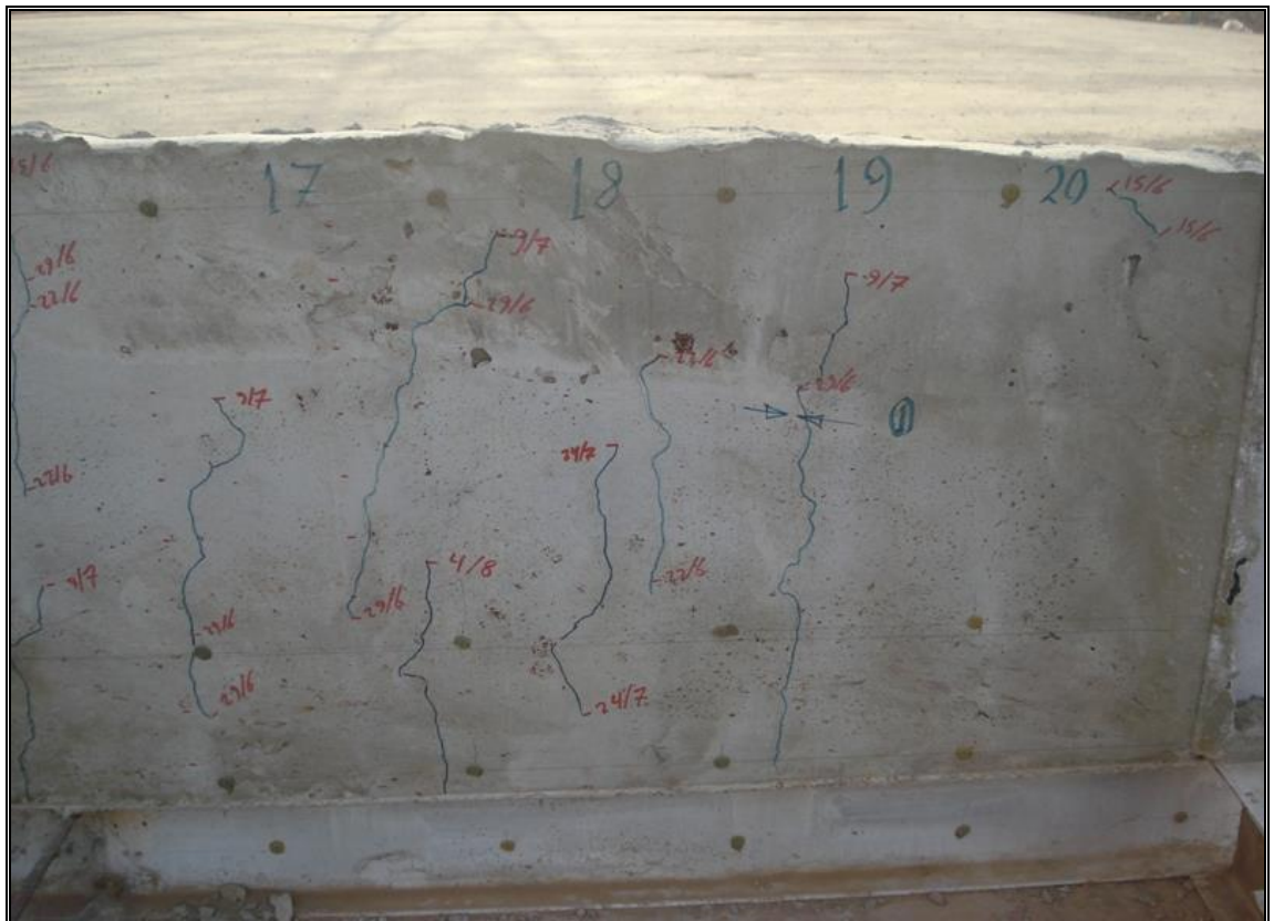
Plate (4-4) Final cracking pattern of fourth quarter of wall (8S)
