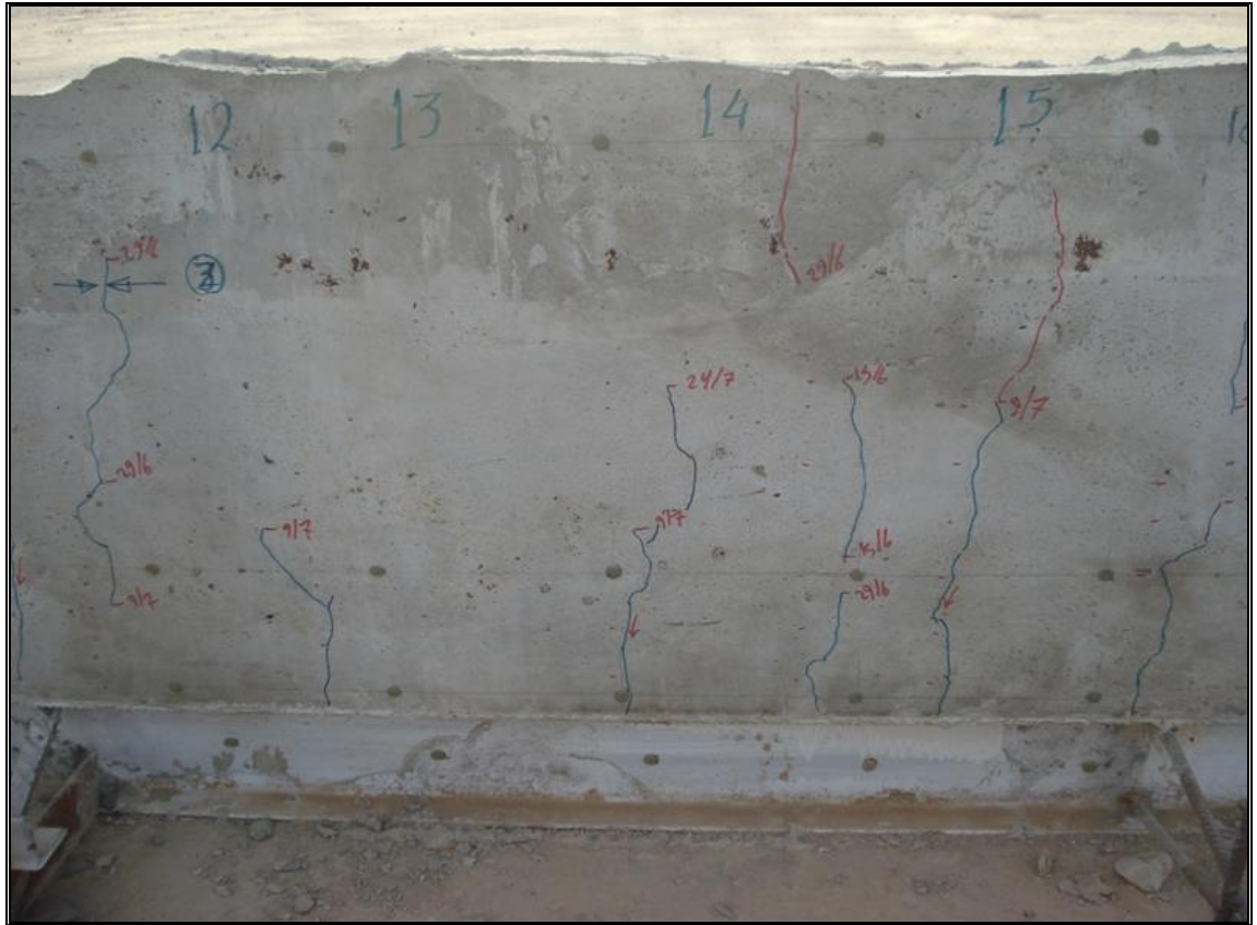
Plate (4-3) Final cracking pattern of third quarter of wall (8S)
