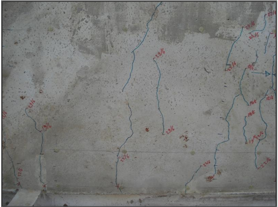
Plate (4-7) Final cracking pattern of third quarter of wall (4S)
