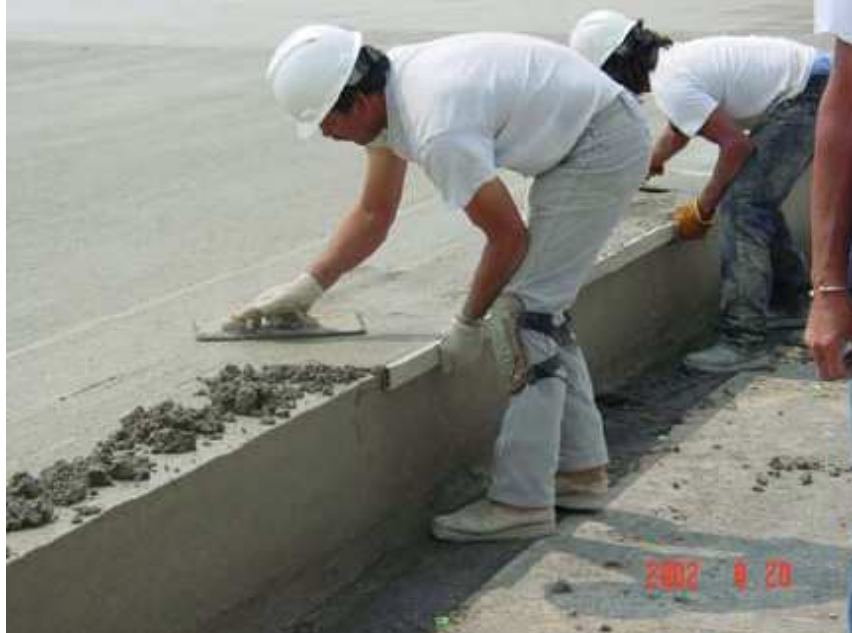
b. Poor practice
