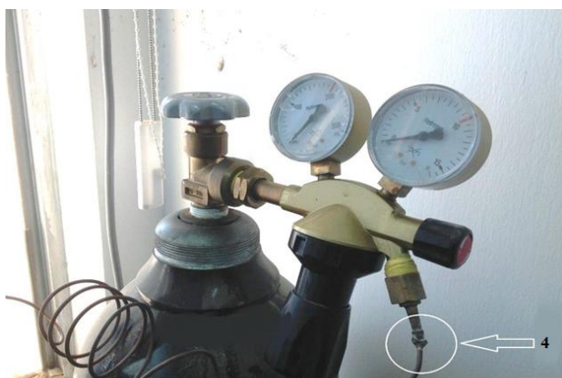
Figure 2. Improperly installed tubing between the gas outlet and the GC, which could lead to hydrogen leaks
