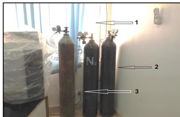
Figure 1. New GC with gas cylinders improperly installed, resulting in a number of safety hazards
