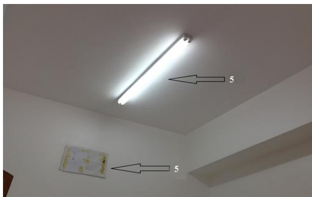
Figure 3. Fluorescent lighting installed in the laboratory and laboratory operating instructions posted too high to be able to be read
