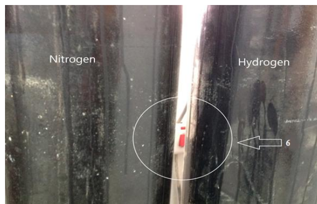
Figure 4. The main switch for the A/C was installed between the hydrogen and nitrogen cylinders
