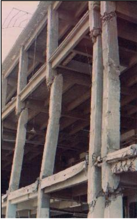
Picture 2. Samples of the columns affected by the substantial damage
