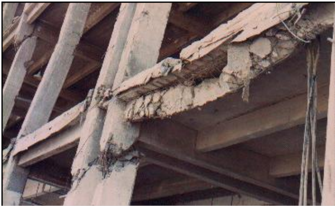
Picture 3. damage occurring from the slab and secondary beams in the slab, located between grids (Y2-Y3/X8-X9)
