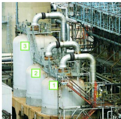
Figure 6 A view of three fixed-bed reactors (Unit 3) which operate in series at an oil refiner. The reforming reaction, which produces aromatic hydrocarbons and hydrogen, takes place in reactor 1, followed by isomerisation reactions in reactor 2 and finally in reactor 3, cracking reactions.
